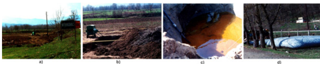
Figure 7. Remediation works conducted at the kerosene contaminated site in Vitanovac in 1994: (a, b), free phase pumping (c), and storage of pumped free phase (d) (Matić, 1994)
